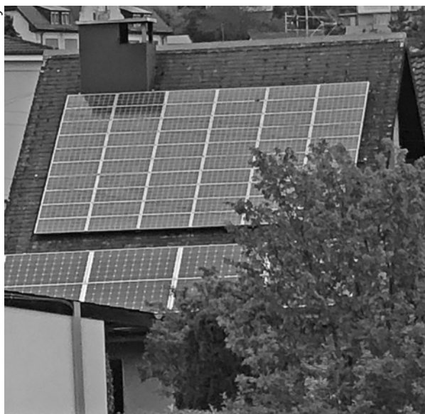
PV Anlage Frey in Niedergösgen
